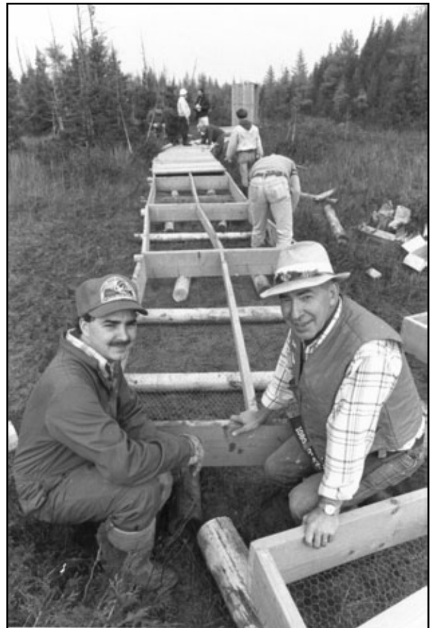
John Morton and Nels Maher pause while building the Oliphant Fen Boardwalk. The official opening of the boardwalk, built to allow visitors to enjoy this habitat without trampling delicate plants, was held in June 1991.
